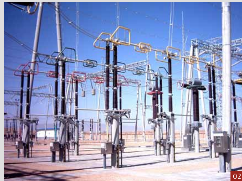
01: 550kV HV Disconnector 02: 363kV HV Disconnector
