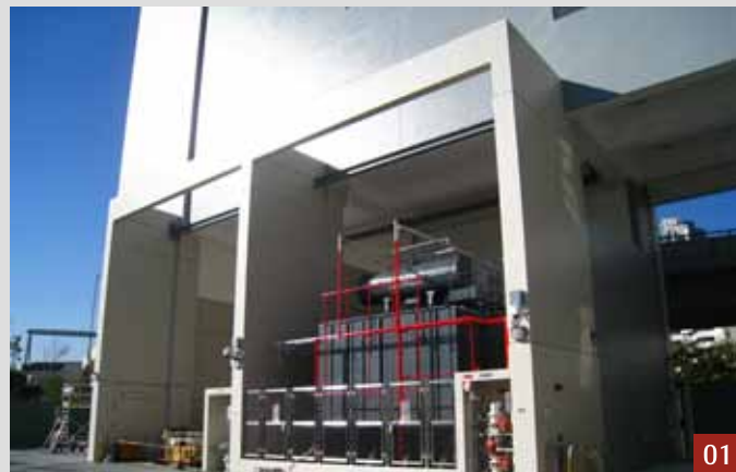
01: 132kV GIS at Junk Bay Road
