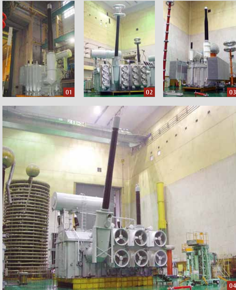
01: 40MVA/1000kV Power Transformer 02: 700MVA/750kV Single-phase Auto-transformer 03: 140MVar/750kV Shunt Reactor 04: 500MVA/750kV Single-phase Auto-transformer
