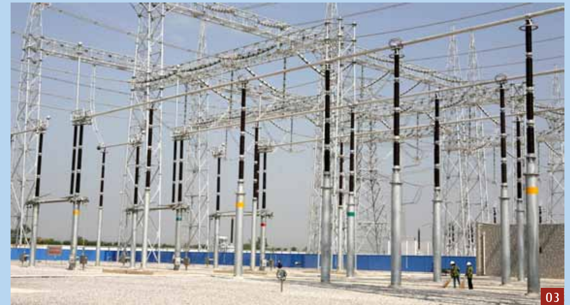
01: 1100kV UHV Disconnecter 02&03: 800kV HV Disconnecter
