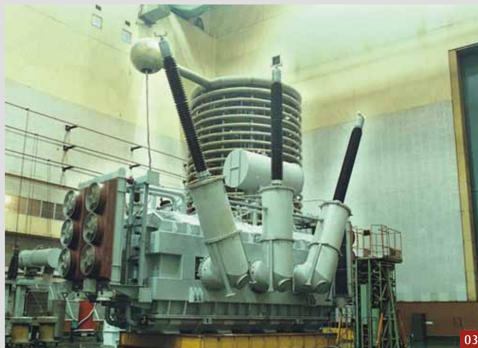
01: 12.6MVA/72.5kV Rectifier Transformer in Canada 02: 60MVar/500kV Shunt Reactor for Fuzhou Power Bureau, China 03: 160MVA/420kV Generator Transformer in Baghdad, Iraq
