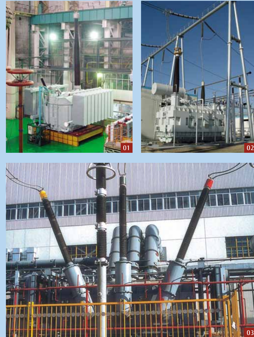
01: 100MVar/750kV Shunt Reactor 02: 250MVA/500kV Auto-transformer 03: 400MVA/500kV Power Transformer in Jungar Banner ,Inner Mongolia
