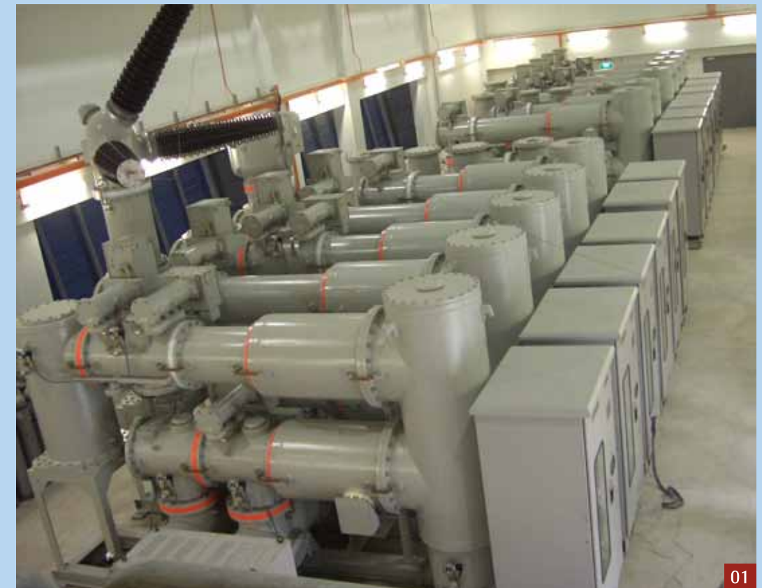
01: 66kV GIS for Nape Substation, in test
